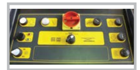
Quadro comando Control panel
